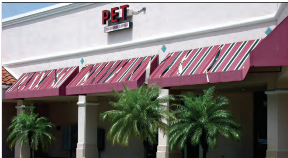
Evidence of Hurricane Isaac's visit to Hobe Sound lies on the shutters of businesses housed in the Winn-Dixie Marketplace Plaza.
