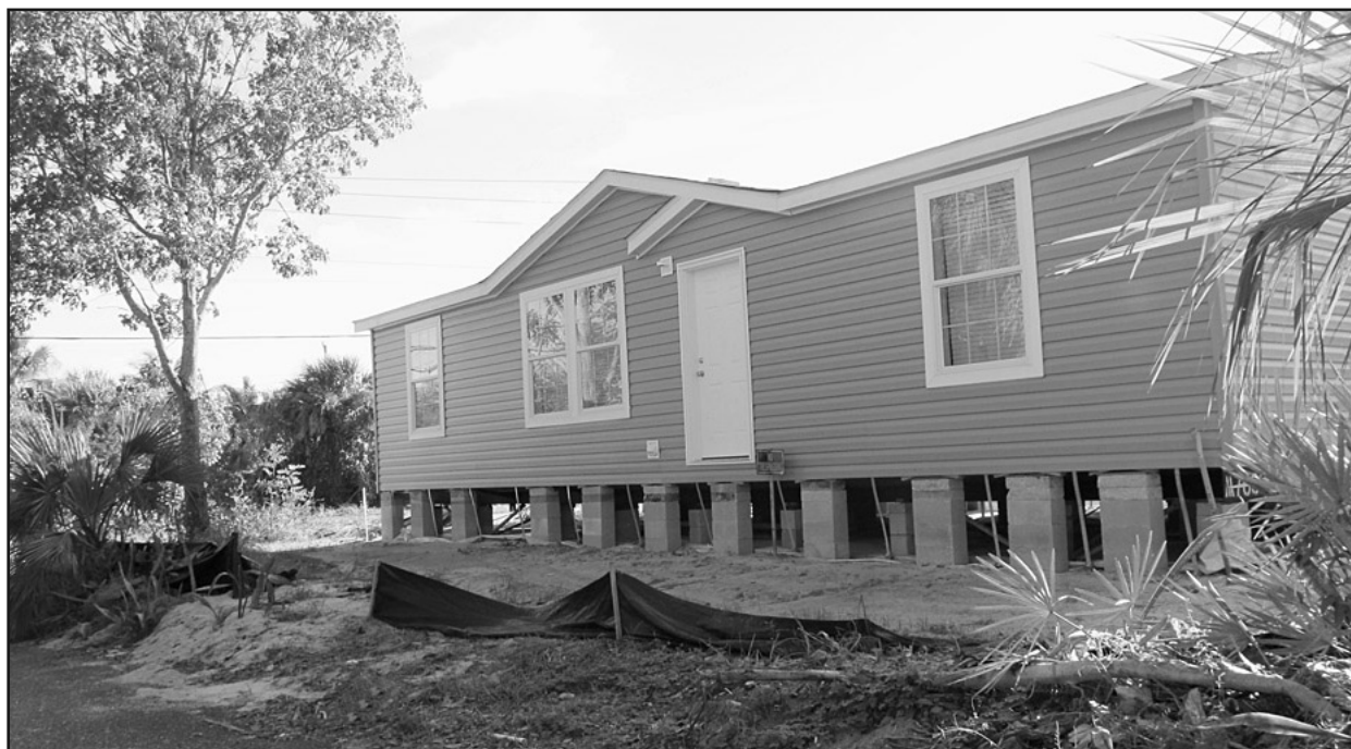
A stop-work order has been placed on the installation of a modular home in the Zeus Park neighborhood of Hobe Sound until the legal issues revolving around its foundation and zoning are settled. The home faces the alley, although its address is on Apollo Street.
